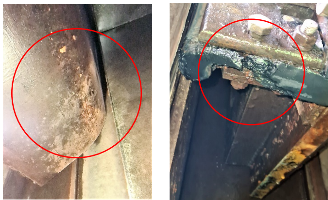
Figure 1. Local damages at the gate bottom (left – gate lip caverns from rock hits, right – side seal bottom face damage)
