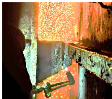
Figure 3. Side bumpers cut-out to release the stuck gate
