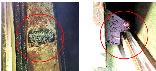
Figure 2. Wheel track damage (left) and side bumper contact with the sliding track (right)
